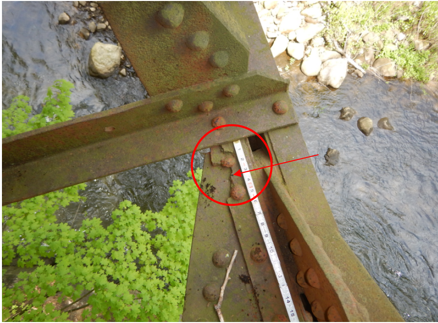
Photo 13: 100% section loss to horizontal angle leg of Span 3, East Truss lower chord member L1L2 at L2, looking down.
