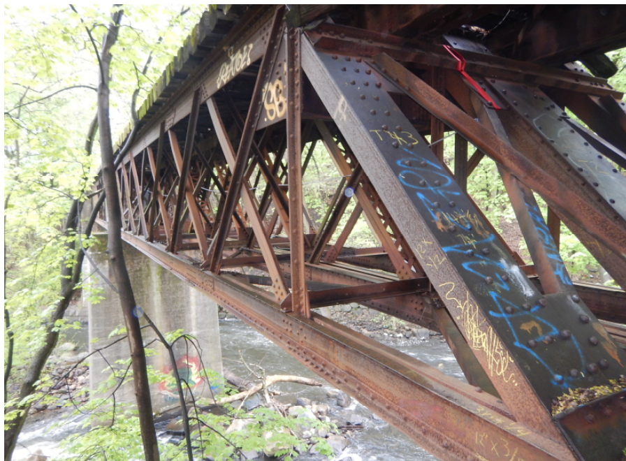
Photo 10: Typical condition of East Truss, Span 3, looking south. Note 100% paint loss with light to moderate corrosion of all exposed steel surfaces. Note graffiti on steel truss members.
