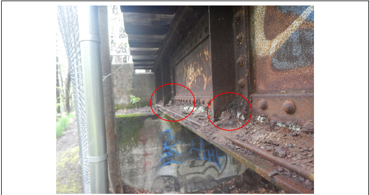
Photo 25: 100% section loss to vertical stiffeners, Span 4, West Girder, looking north. Note heavy debris on girder bottom flange.
