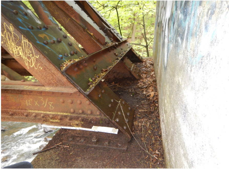
Photo 11: Severe corrosion and section loss with hole in angle leg at Span 3, East Truss, lower chord member L7L8 at L8, looking west on Pier 3.
