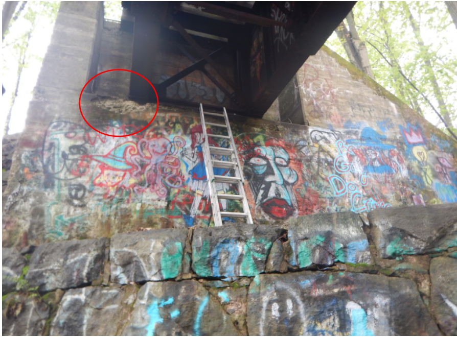
Photo 27: Spall in South Abutment seat, looking south. Note heavy graffiti on abutment breastwall.
