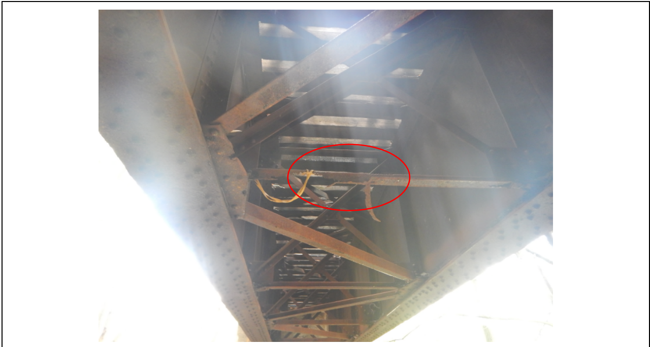
Photo 23: Underside of Span 1 deck girders, looking north. Note severe corrosion to horizontal cross bracing.
