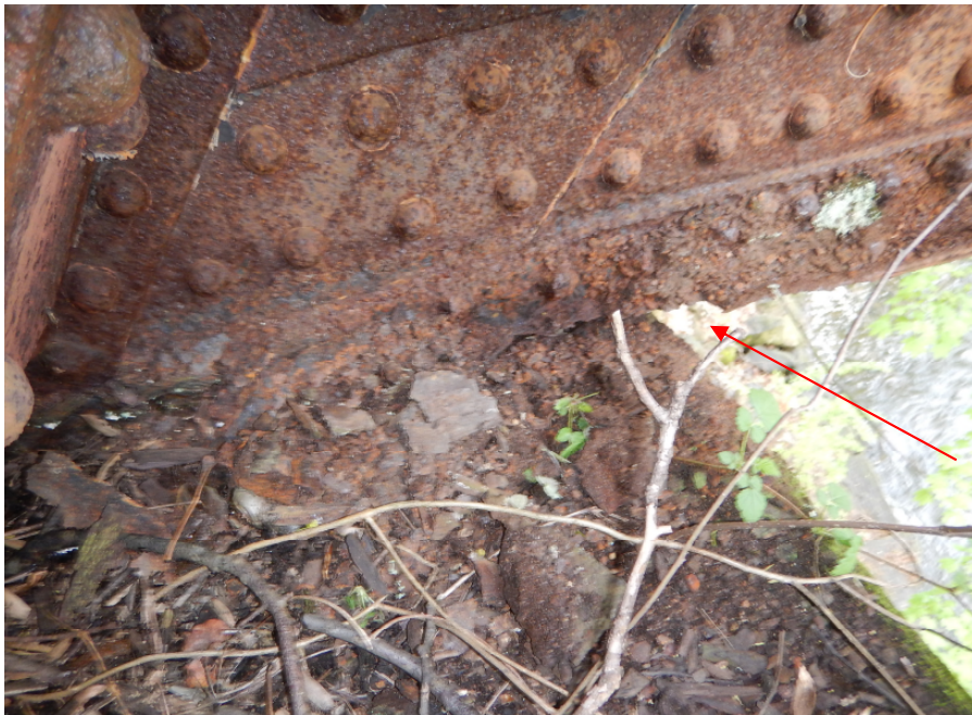
Photo 14: 100% section loss to horizontal angle leg of Span 2, Center Truss lower chord member LOL1 at L0, looking west. Note heavy debris around bearing.
