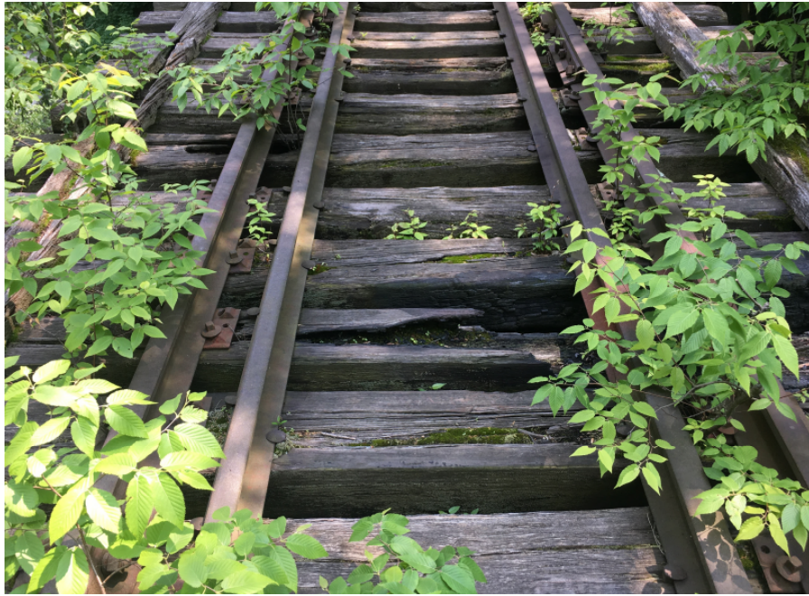
Photo 9: Fire damage to timber ties, note heavy vegetation growth, typical throughout all spans, looking south.
