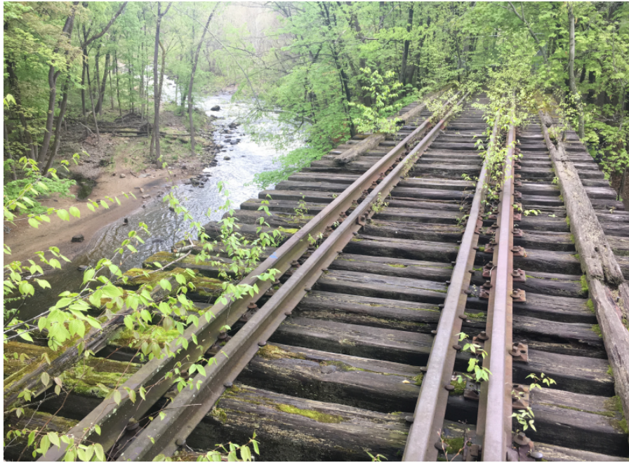
Photo 7: Typical top of deck condition, severe rot and decay of timber ties with heavy vegetation growth, looking northwest.
