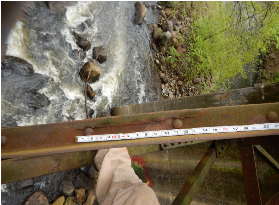
Photo 12: 13" long crack in horizontal leg of Span 3, East Truss diagonal member L3U2, looking down.
