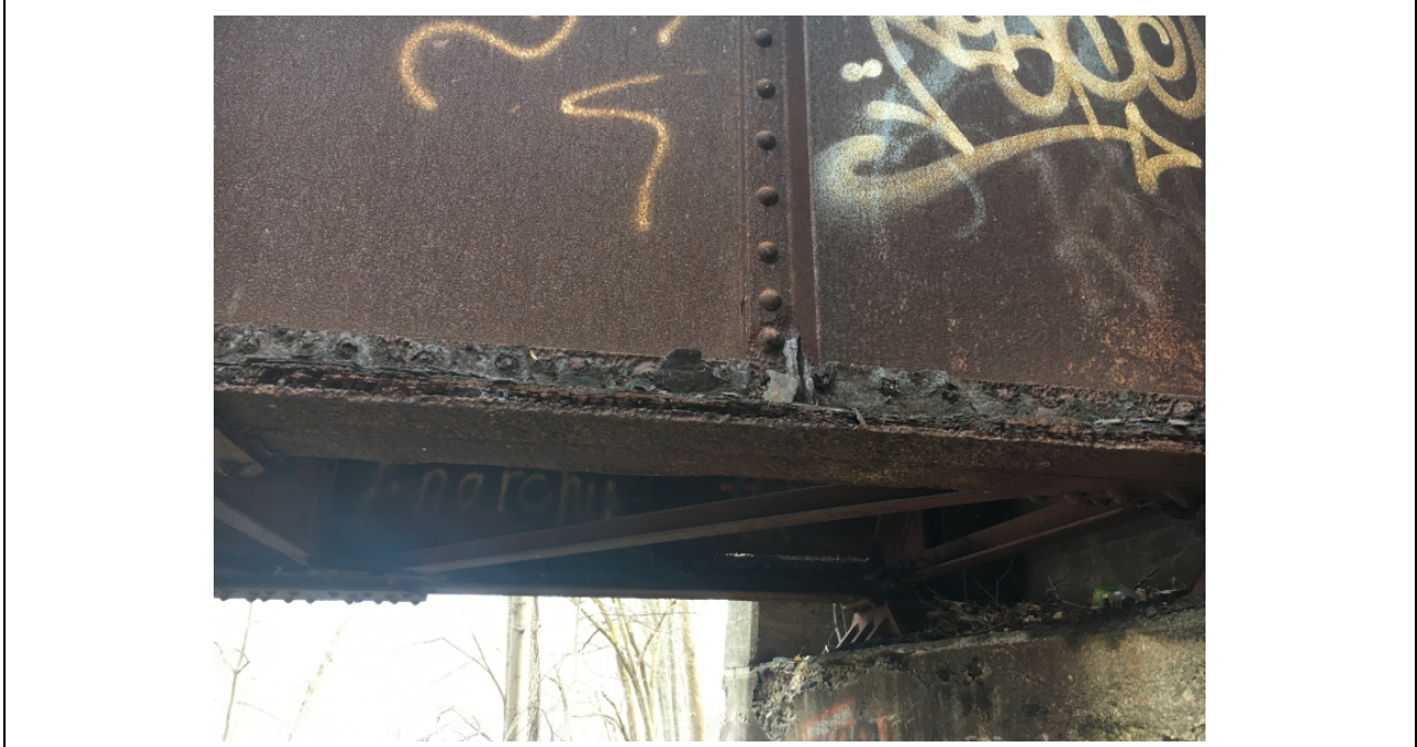
Photo 24: Severe corrosion to bottom flange angles, Span 1, West Girder, looking east.
