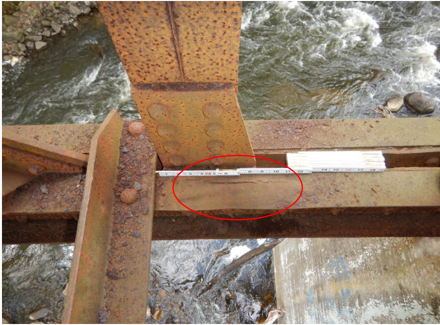
Photo 17: 10" long crack in horizontal leg of Span 2, West Truss lower chord member L7L8 at L7, looking west.
