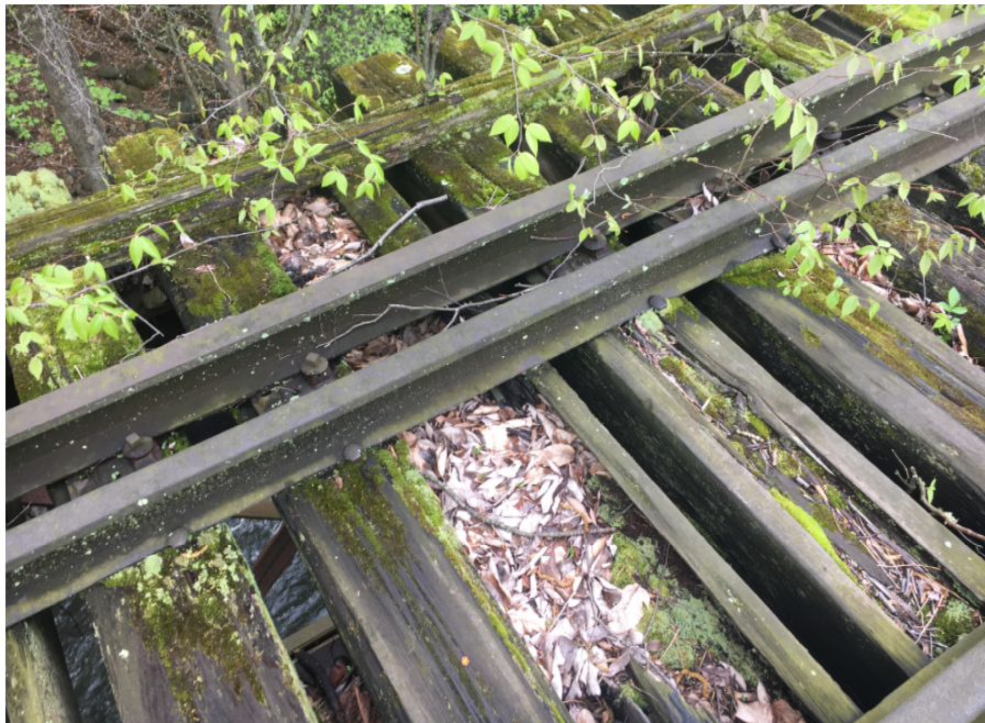
Photo 8: Severe rot and decay of timber ties, typical throughout all spans, looking west.
