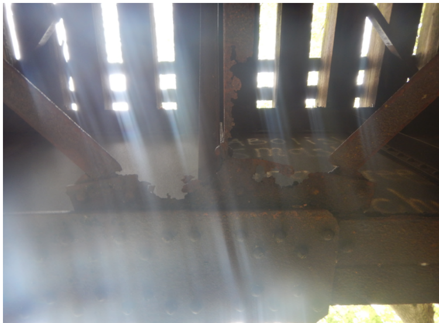
Photo 22: Severe corrosion and 100% section loss to lower horizontal bracing members, Span 2 at West Girder, looking west.
