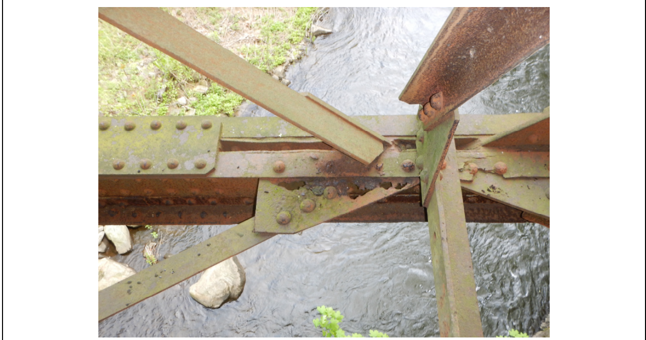
Photo 20: 100% section loss to truss lower horizontal bracing at Span 2, East Truss L2, looking down.
