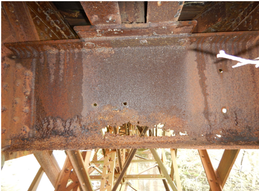
Photo 18: Large web hole and lower flange section loss at end floorbeam at U1, Span 2 between Center and West Trusses, looking north.
