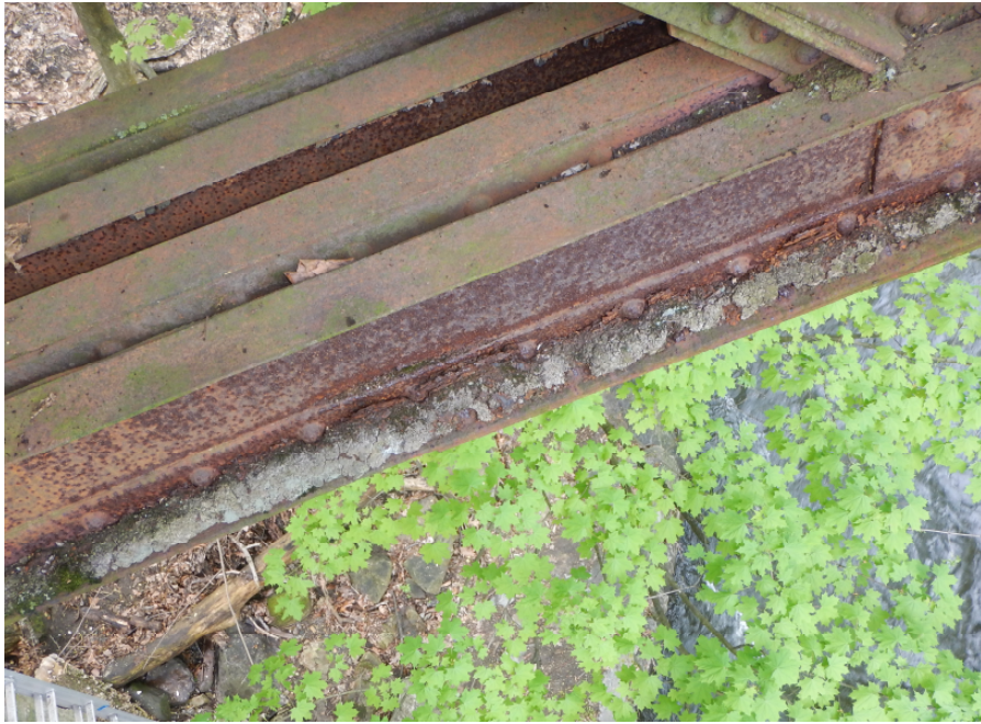
Photo 15: Severe corrosion and section loss to Span 2, Center Truss lower chord member L1L2, looking down.
