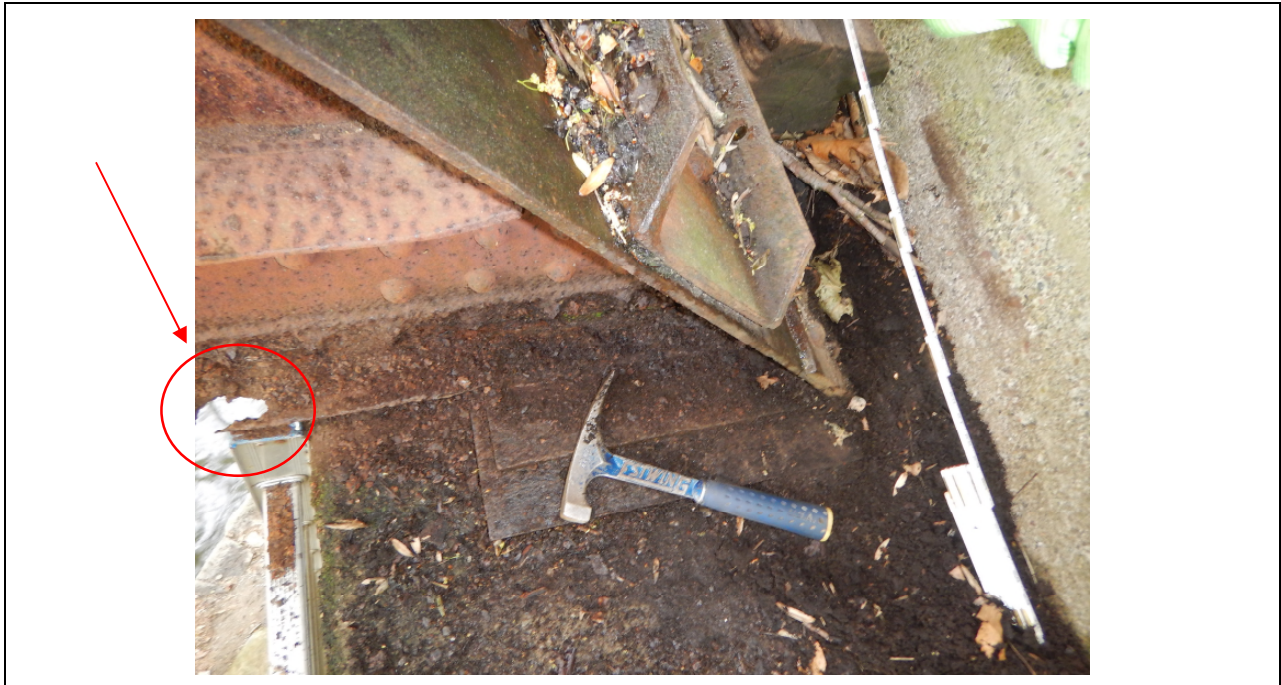
Photo 19: Heavy dirt and debris accumulation at truss bearing over Pier 1, looking west. Note large hole in lower chord member L0L1 at West Truss.
