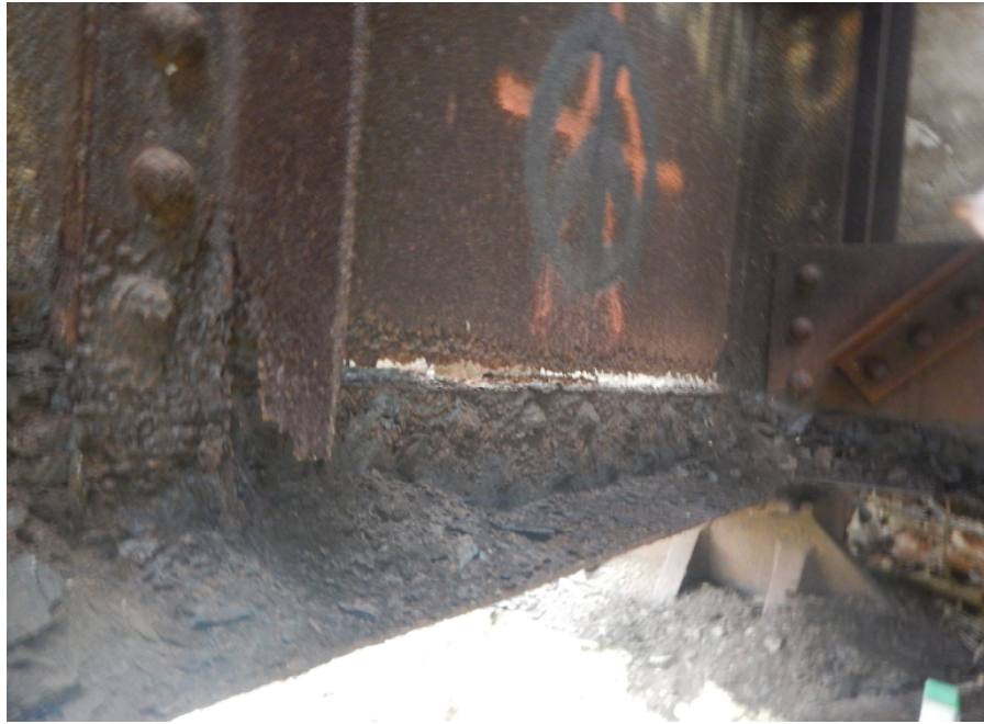
Photo 21: 100% section loss and holes in girder web and vertical stiffeners, Span 1 East Girder at South Abutment, looking southeast.
