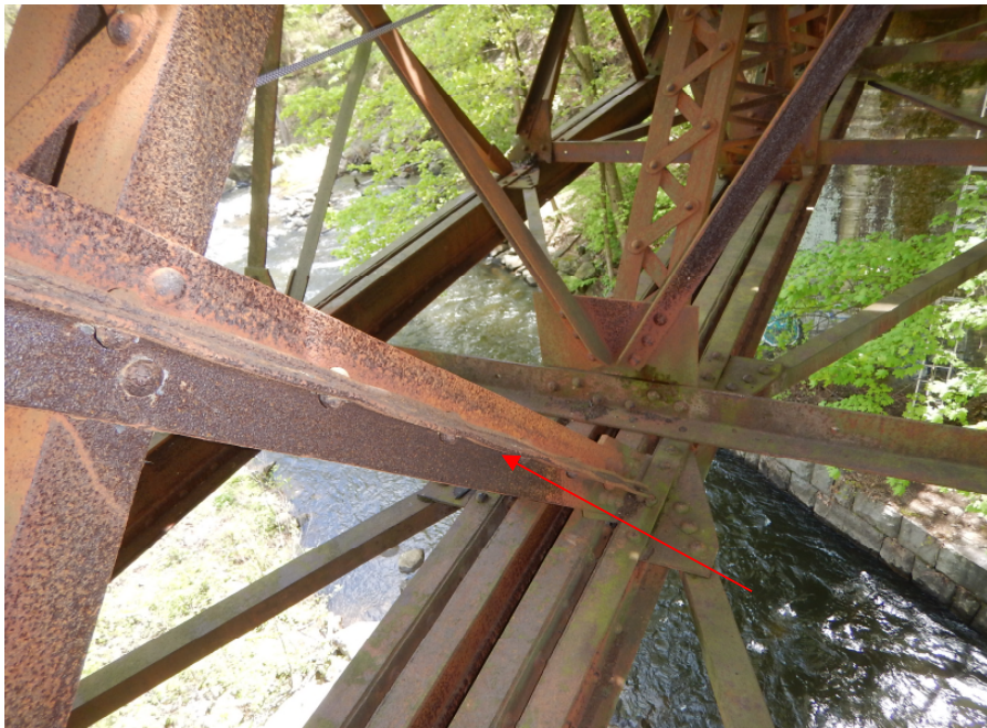
Photo 16: Typical condition of truss members, Span 2 Center truss, looking north. Note pack rust between riveted angles.
