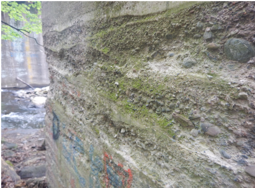
Photo 28: Heavy scaling to west face of Pier 1, looking north.
