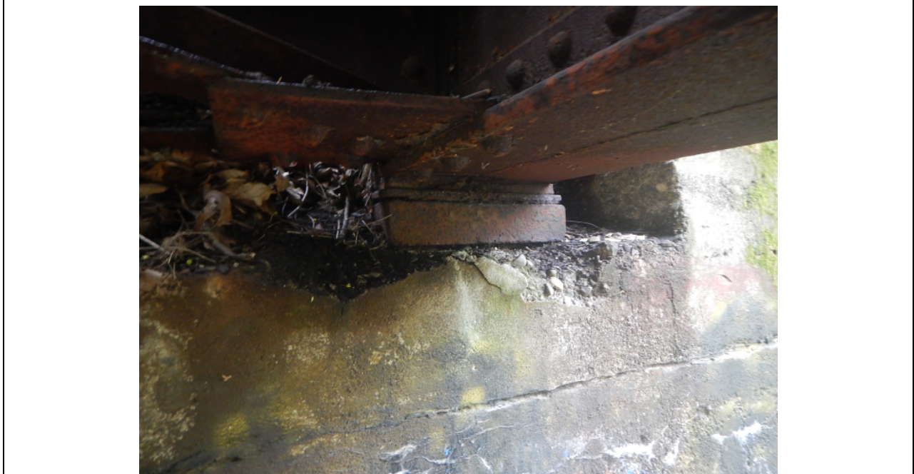
Photo 26: Large spalls in Pier 3 seat below girder bearing, looking south.
